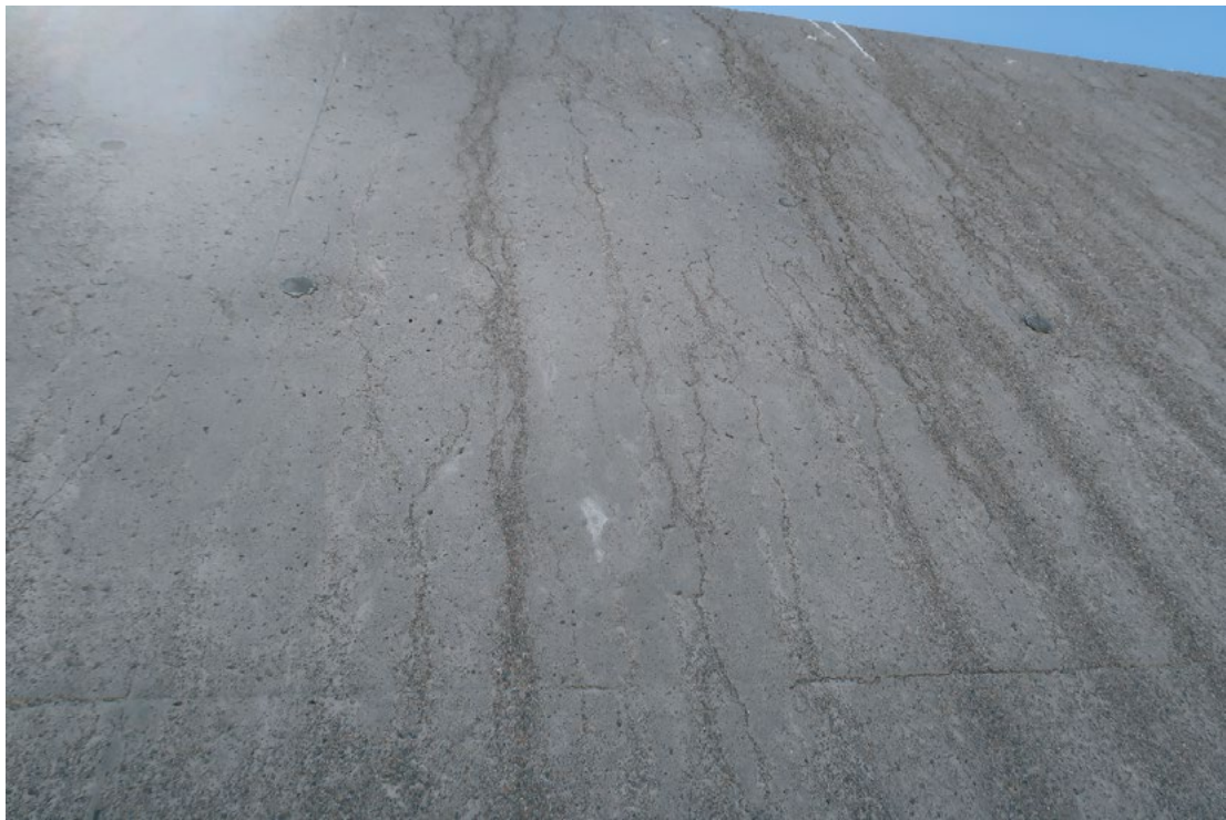
Compaction defects in the concrete cover (surface trails).
