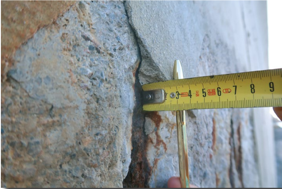
Advanced corrosion due to lack of cover.
