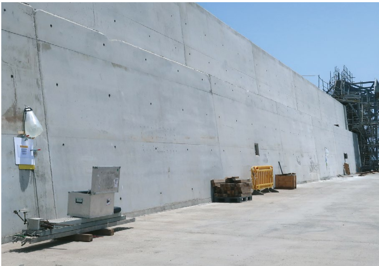
Study of corrosion in the reinforced concrete of the Reina Sofía dock, in the port of Las Palmas.
