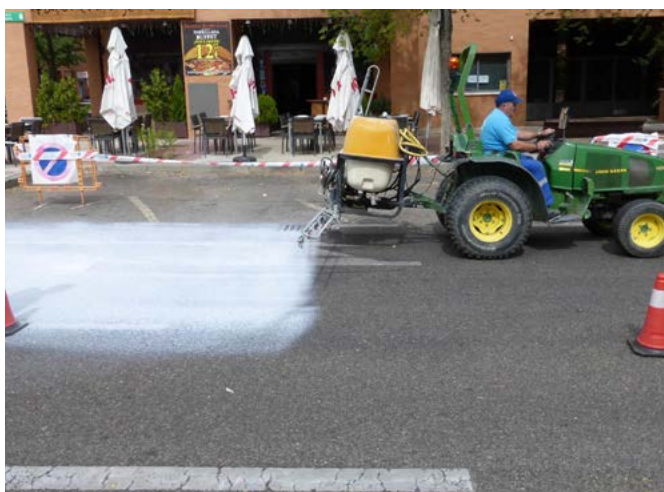
Application of the photocatalytic product on the surface of the Paseo de la Chopera road in Alcobendas
