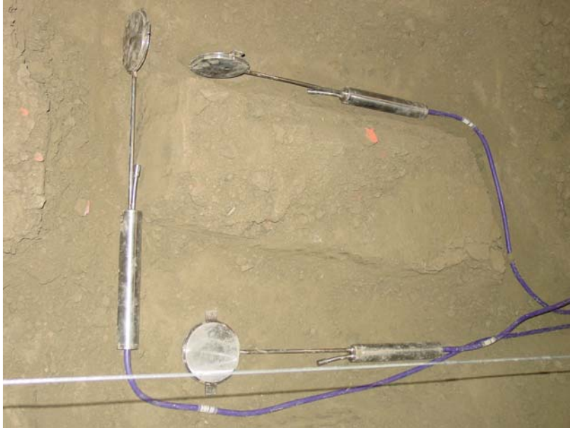
Figure 8. Triaxial set of Geokon® stress cells in the subgrade.
