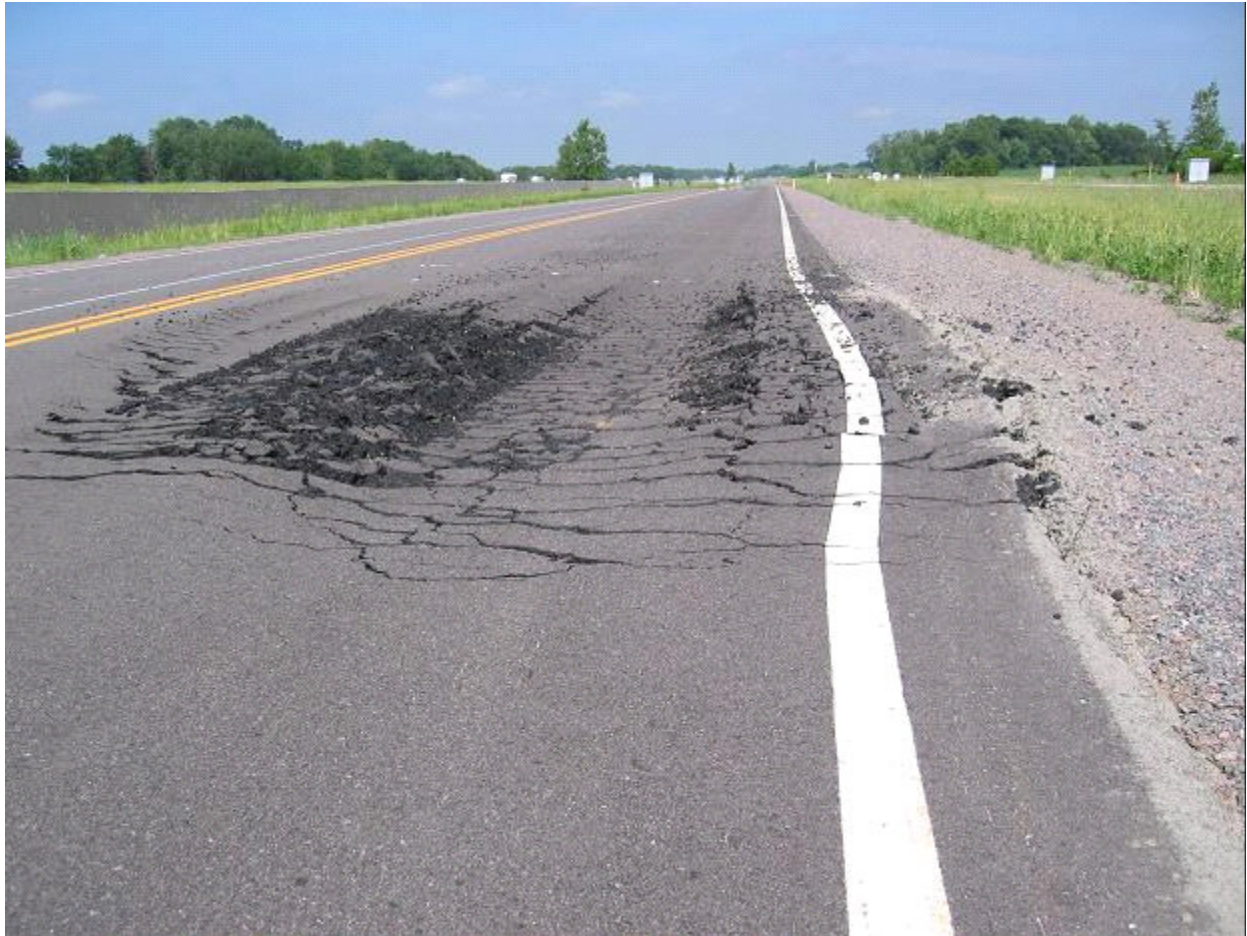
FIGURE 9 Condition of Cell 28 Before Forensic Investigation.
