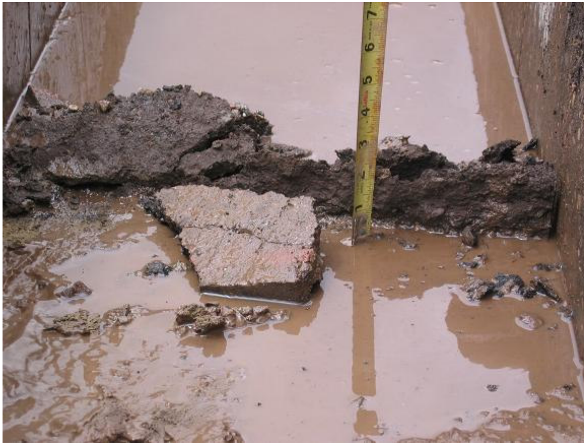
FIGURE 5 Ridge of Pumped Fine Material at Transverse Crack Face.
