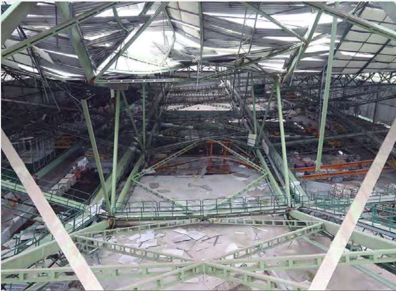
← Laboratory hall's collapsed structure.
