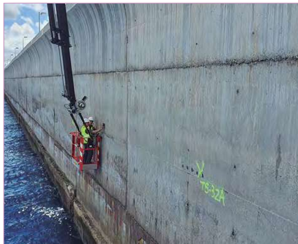
Research of corrosion in the reinforced concrete of the Reina Sofía Dock (port of Las Palmas).
