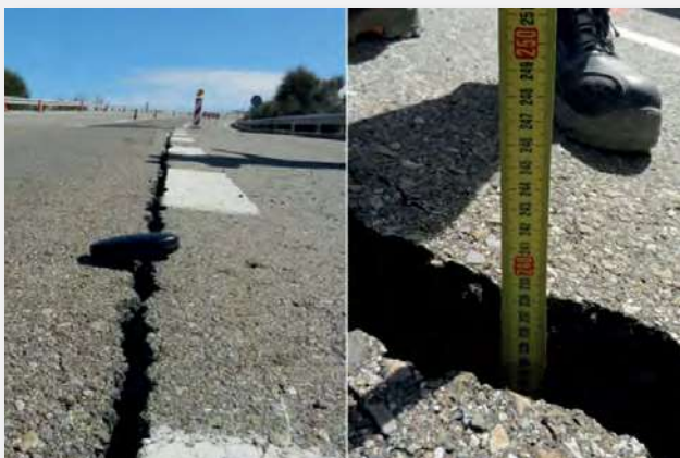
↑ Cracks in the pavement.
