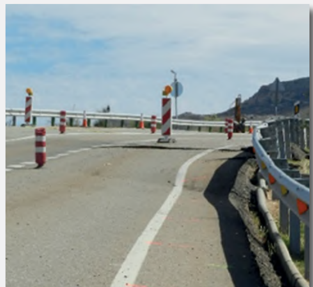
↑ Deformation of the road surface.
