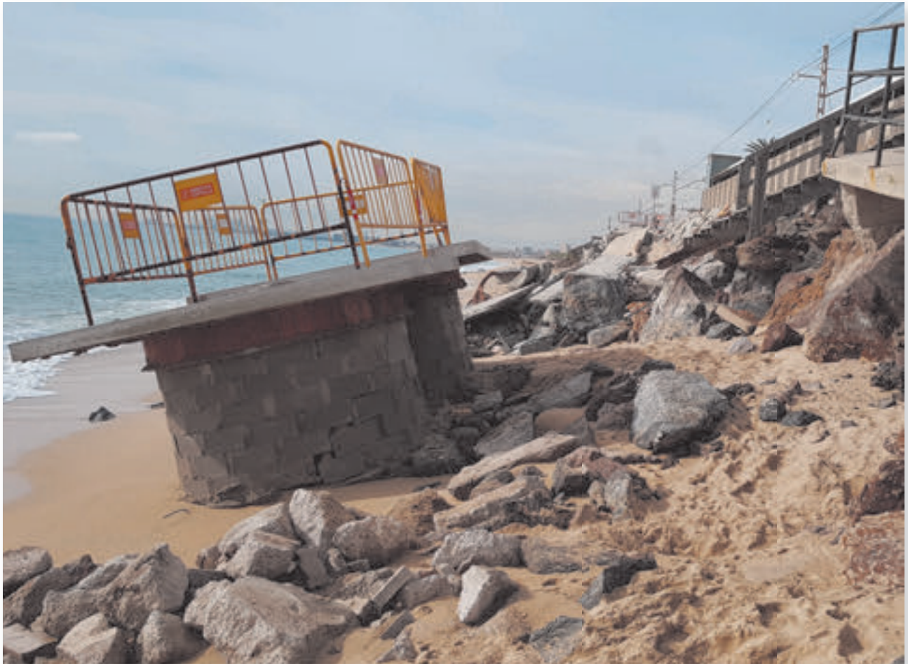
View of the beach erosion and seawall collapse, Mongat (Barcelona) after the storm Gloria.
