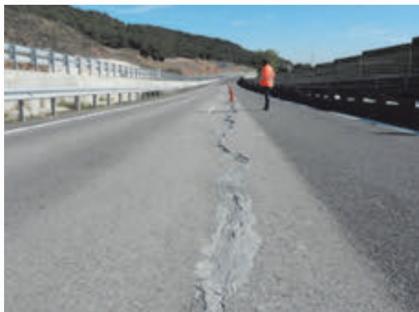
Cracks on the pavement of right carriageway.
