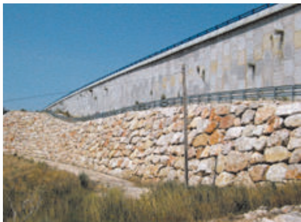
View of the hybrid wall (reinforced soil and rock) next to the BU-30 right carriageway.
