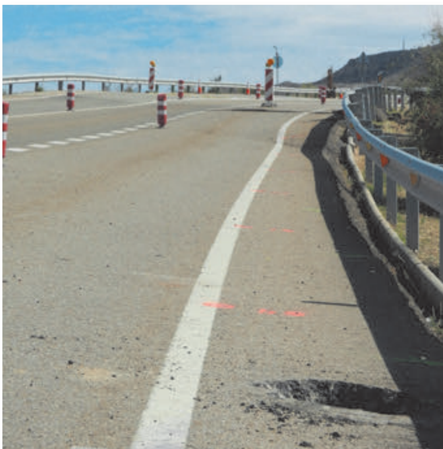
Figure 1. Study of geotechnical road pathologies for the DGC. Bypass of Escucha (Teruel).
