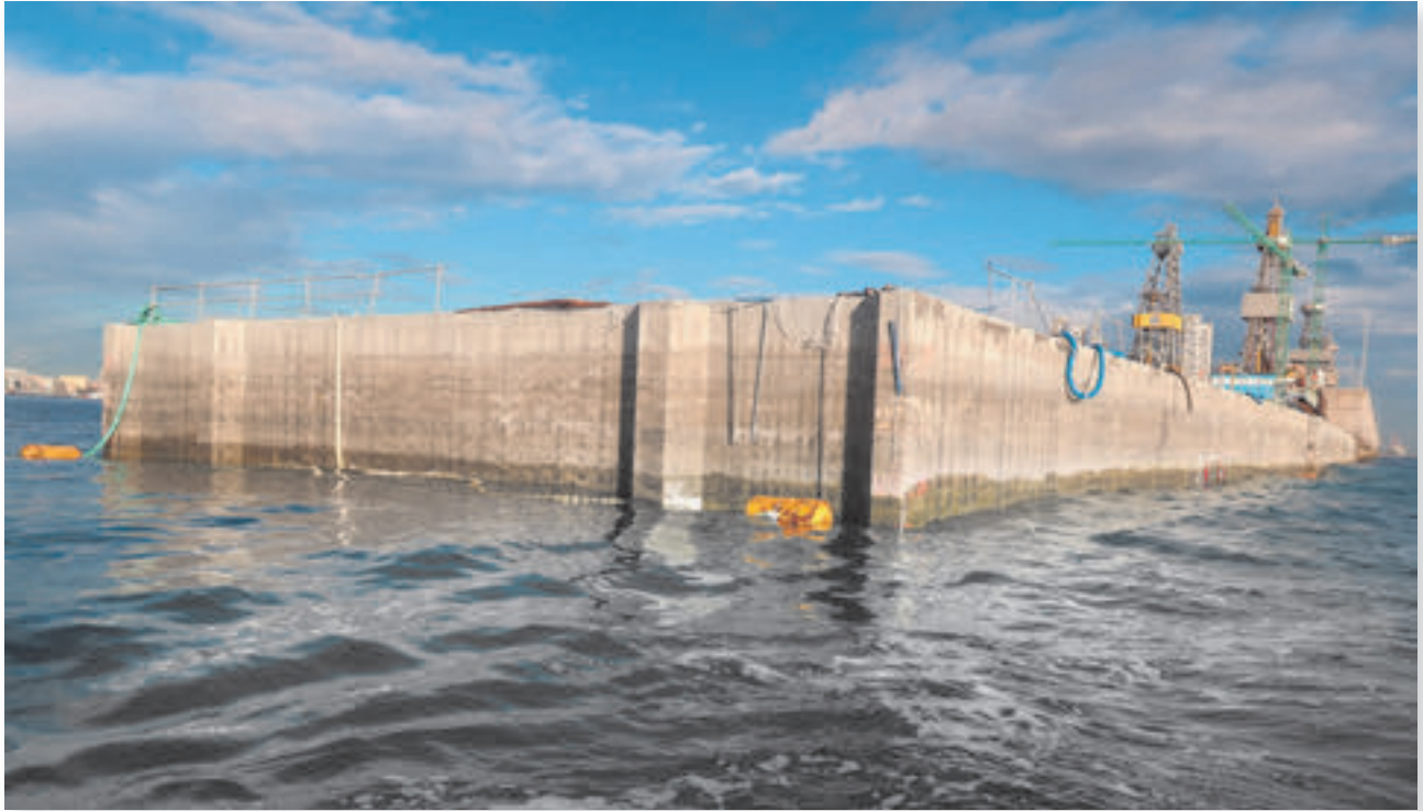
Caisson at anchor in the works of enlargement of Reina Sofía dock, port of Las Palmas de Gran Canaria.
