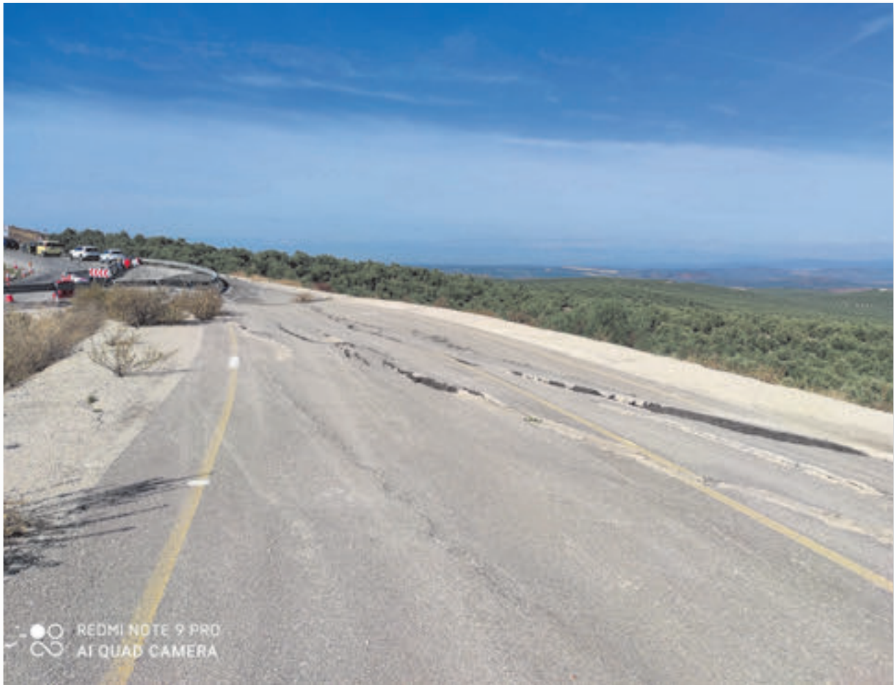
Figure 2. Studies of geotechnical damages on roads. Link of Canena (Jaén).
