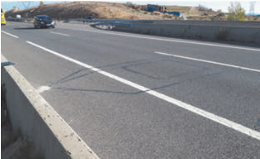
Figure 2. Appearance of the weight sensors and the induction loop installed on the road. Technician of the installation company checking the electronic equipment housed in an outdoor cabinet, next to the solar panel for electricity supply.
