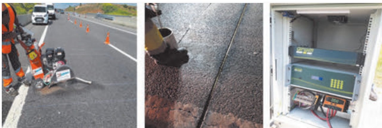
Figure 1. Execution of the pavement cut with a diamond blade saw to excavate the grooves where the sensors are inserted. Appearance of the piezopolymer sensor in the groove. Cabinet that houses the electronic equipment that governs the operation of the WIM system.
