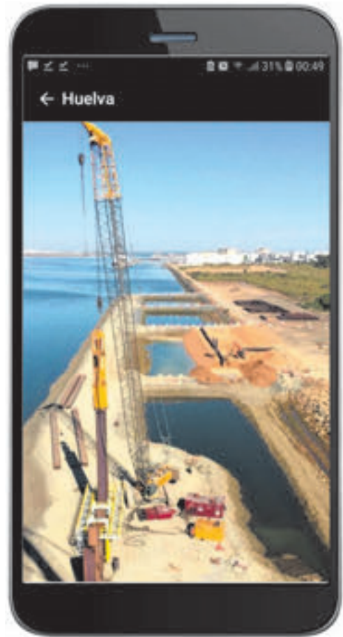
Figure 4. Expansion of the southern pier of port of Huelva, by means of sheet pile walls.
