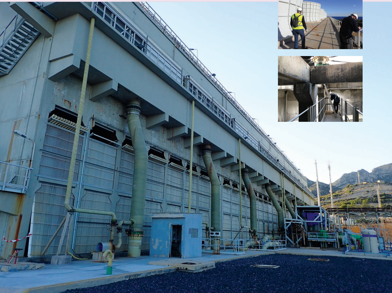
Inspection of the cooling towers of the combined cycle power plant of Plana del Vent.
